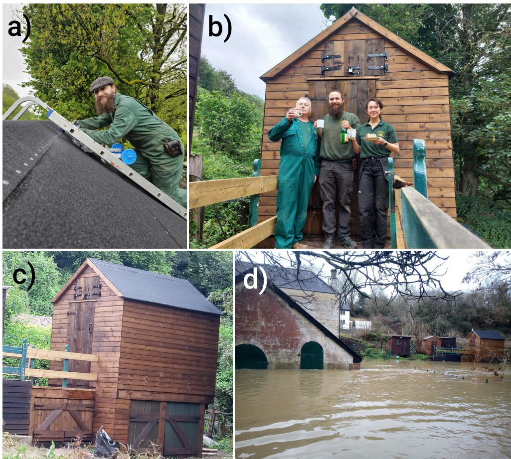
Figure 3: a) Volunteer Julian Stirling finishing the roof. b) Volunteers Steve Denning, Julian Stirling, and Soo-Hwa Kim celebrating topping out. c) The completed building with undercroft storage for items that are not affected by floods. d) The raised outbuildings above a flood that has inundated the pumphouse.
